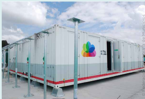
Smart Cloud data centre
